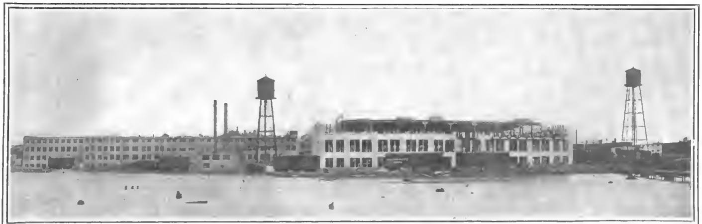
The new addition to the KisselKar plant at Hartford, Wis., will be under cover in thirty days.
